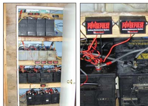
(Top) Larry Sunell uses two large solar panels to charge the battery bank (below left) on his cabin in Canada. A set of PowerPulse units (below right) helps keep the batteries clean so they can accept, store and release a full charge all the time.
